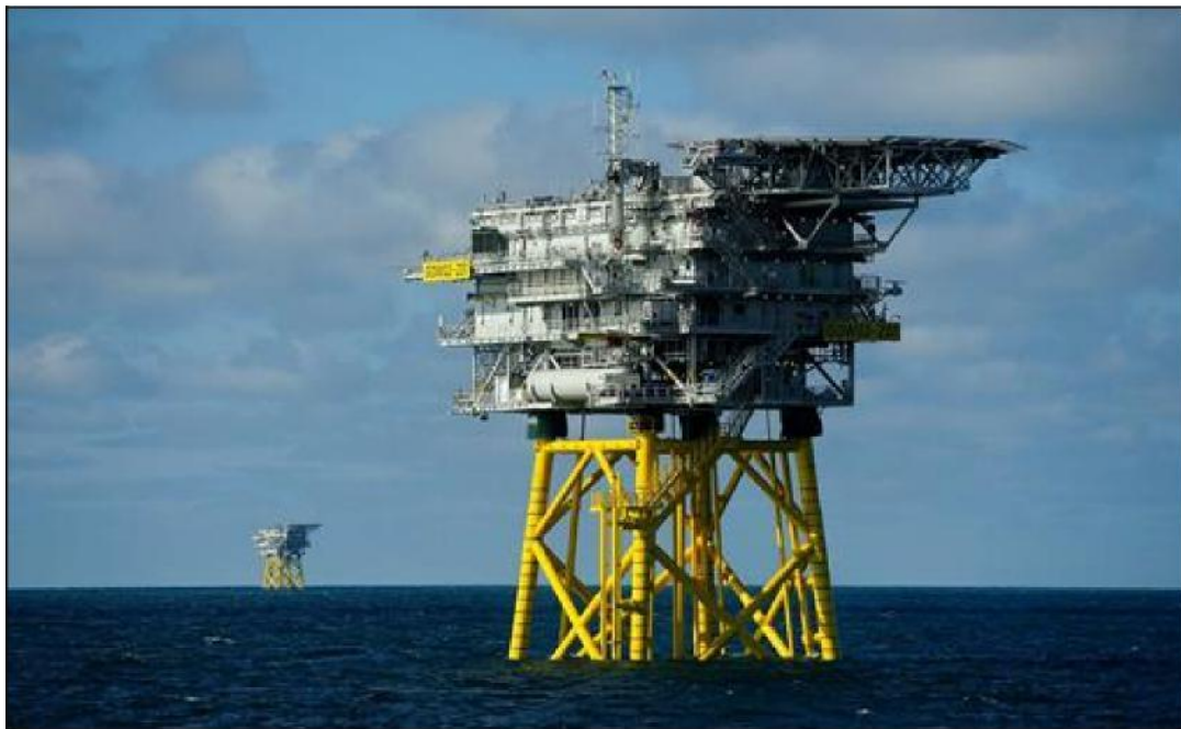
Figure 4.6: Offshore substations at Gode Wind offshore wind farm.
